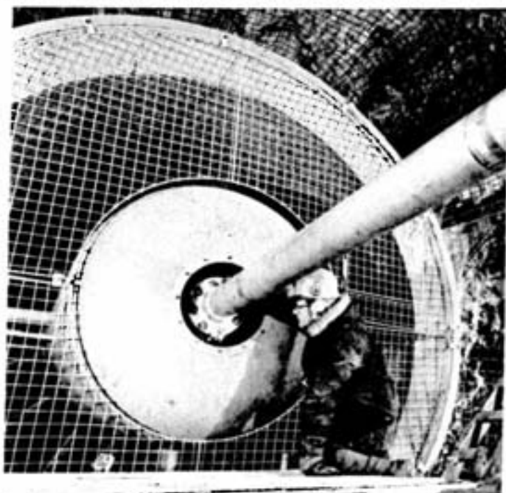
Art Bradbury, a maintenance mechanical leader, checks the shaft lineup, ensuring that the shaft is properly centered and the bolts are properly tightened. Even the slightest deviation will cause excessive vibration, resulting in rapid bearing wear.
